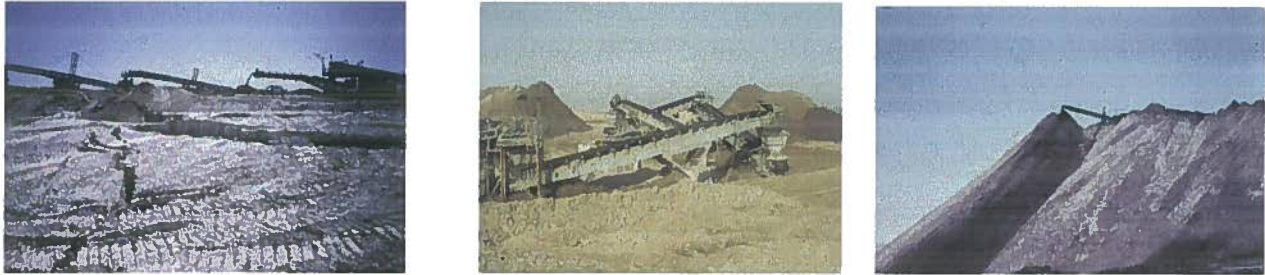
Fig 9 (a) Cracks in dry stack on level ground; (b) Dry stacking using grass hoppers; (c) Advancing face of dry stack
