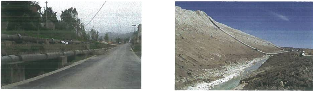
Fig. 1. (a) High pressure gypsum slurry pipelines; (b) HDPE slurry line to stack top
